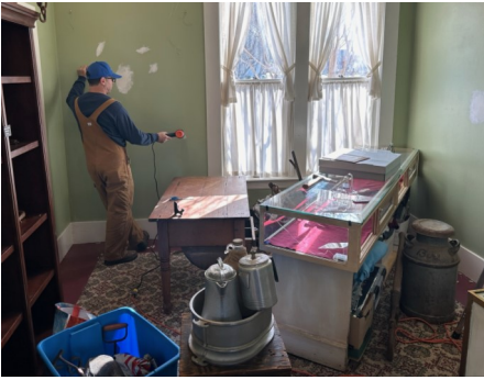
Above: Between exhibits, repairs are made to the walls for a new exhibit. Here, Raul Campos uses his professional expertise to restore the walls in preparation for the Her Story exhibit.
